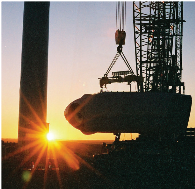
Wind turbine nacelle installation. The nacelle weighs about 110,000 pounds and is the size of a school bus. (Courtesy of Barnhart Crane & Rigging).
