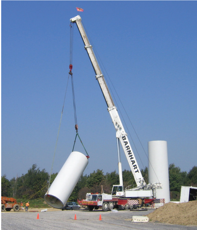
A state-of-the-art rigging system allows a single crane to pickup an angled load that usually requires two cranes. [Courtesy of Barnhart Crane & Rigging].
